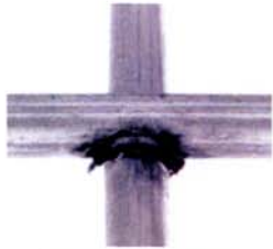
Other wire mesh is zinc galvanized before welding (GBW) - the weld has no zinc, causing premature rusting in any environment
